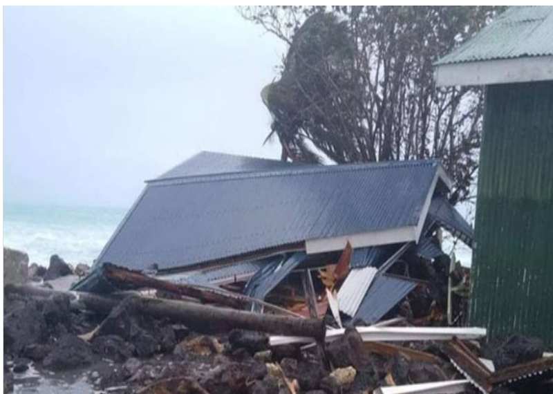
Figure 19: Oinafa Jetty in Rotuma damaged as a result of storm surges and damaging winds on January 17 th . Picture credit: Fijivillage.
